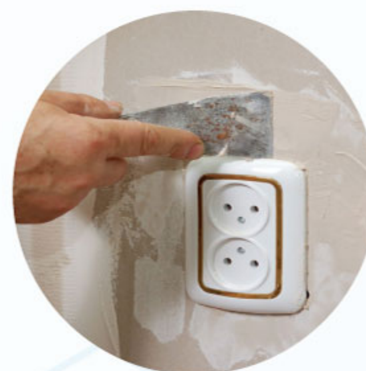
GAP AROUND POWER OUTLET
