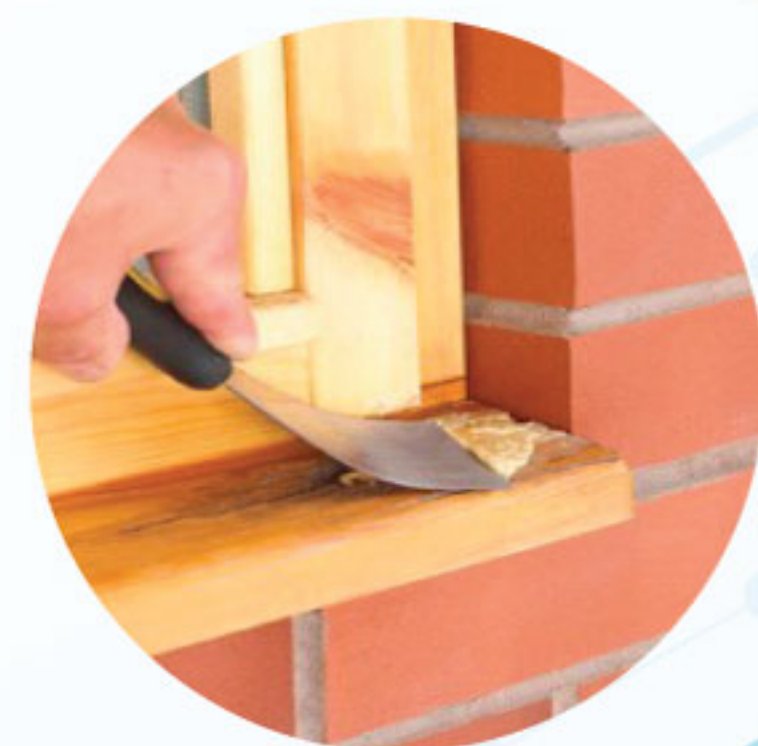
WOODEN FRAME GAP
