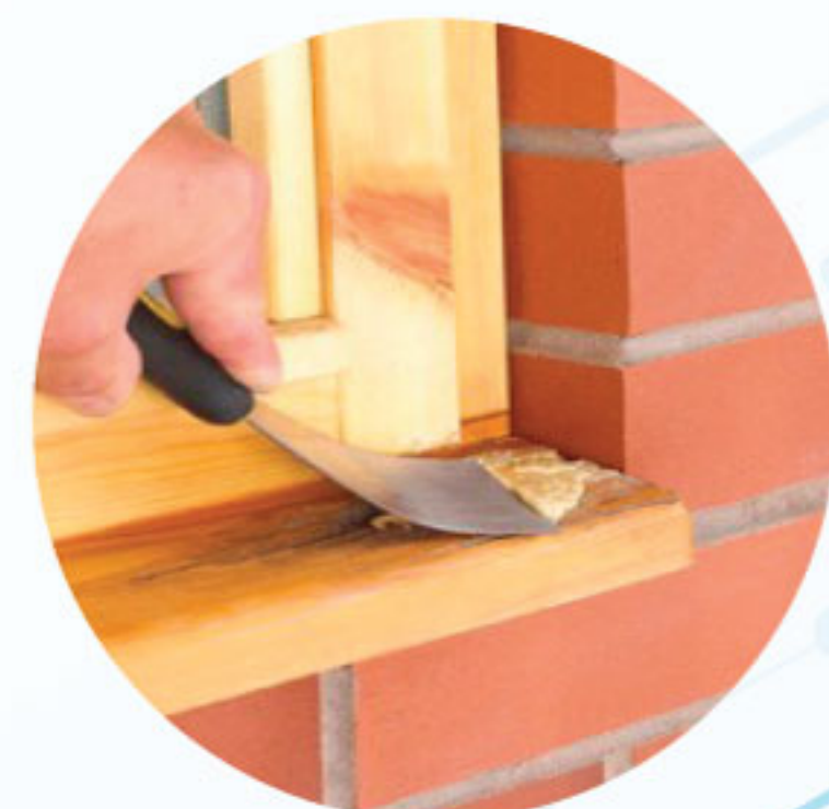
WOODEN FRAME GAP
