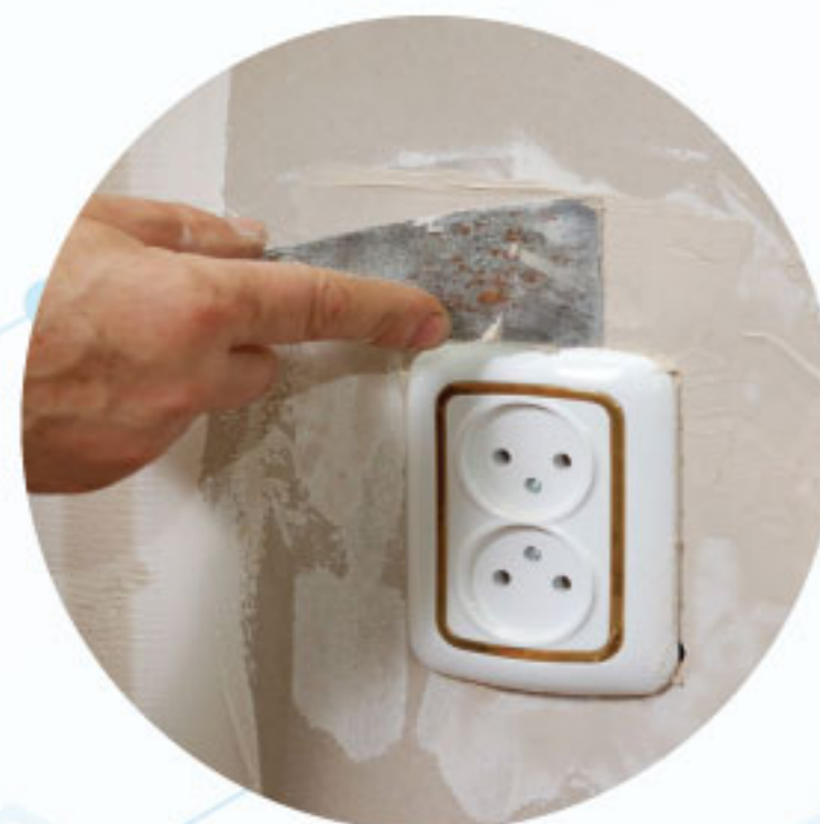
GAP AROUND POWER OUTLET
