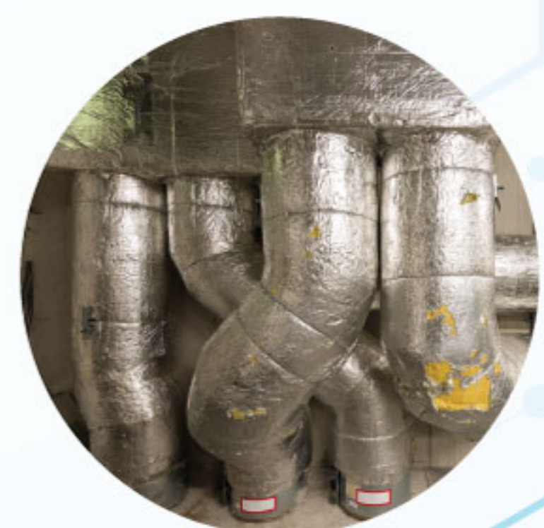
INSULATION FOR DUCTS & PIPES
