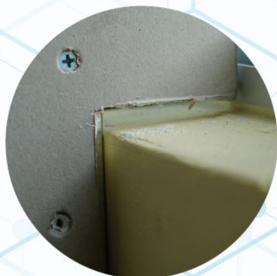
PARTITION TO WALL GAP
