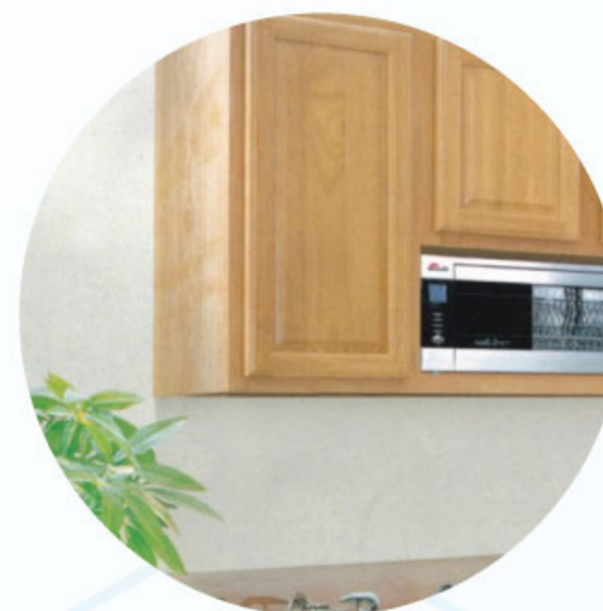
GAP BETWEEN WALL & CABINET
