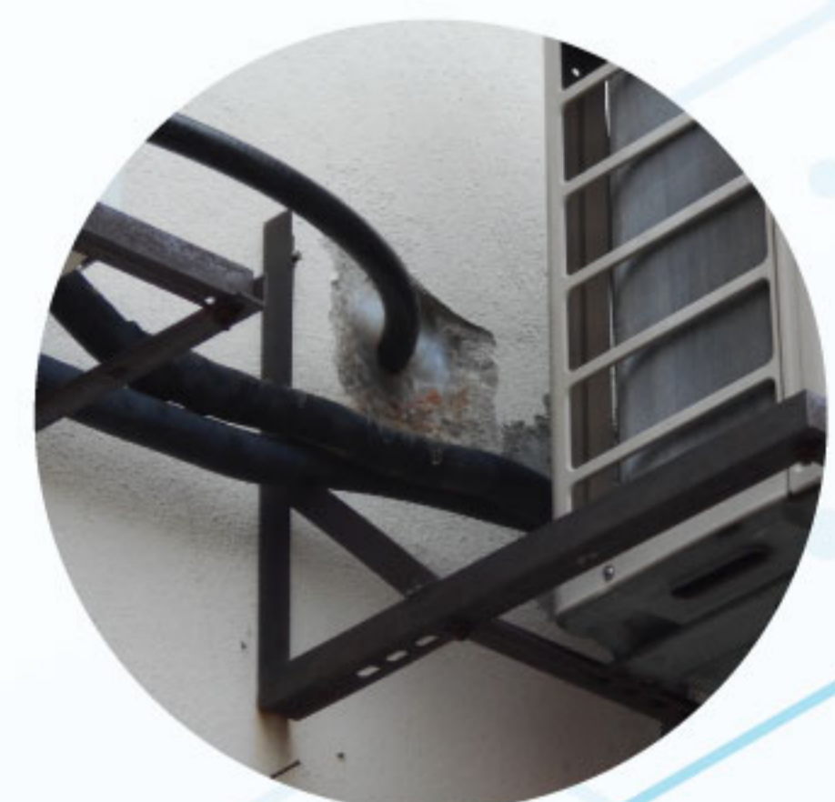
PENETRATION GAP SEALING
