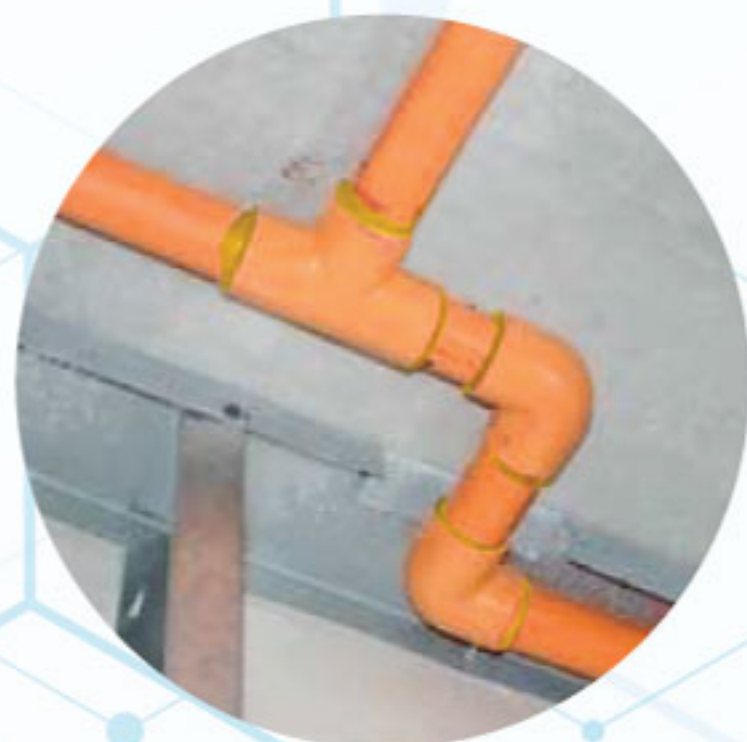
FIRE SPRINKLER PIPES
